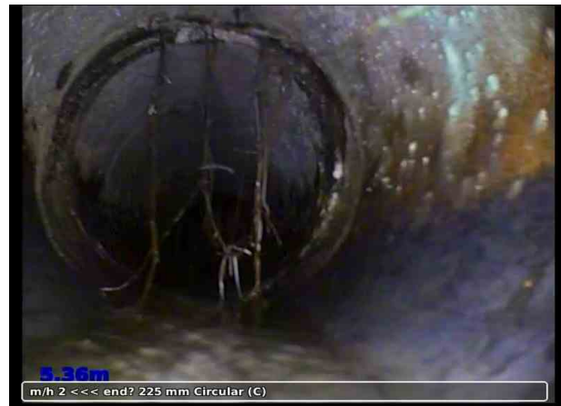
4, 00:02:07, 5.36 m Roots, fine at joint
