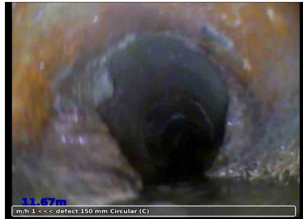
6, 00:01:28, 11.70 m Attached deposits, encrustation from 6 o'clock to 9 o'clock, 10% cross-sectional area loss
