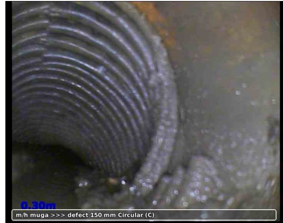
2, 00:00:44, 0.30 m Pipe material changes to an unidentified type of plastic at this point
