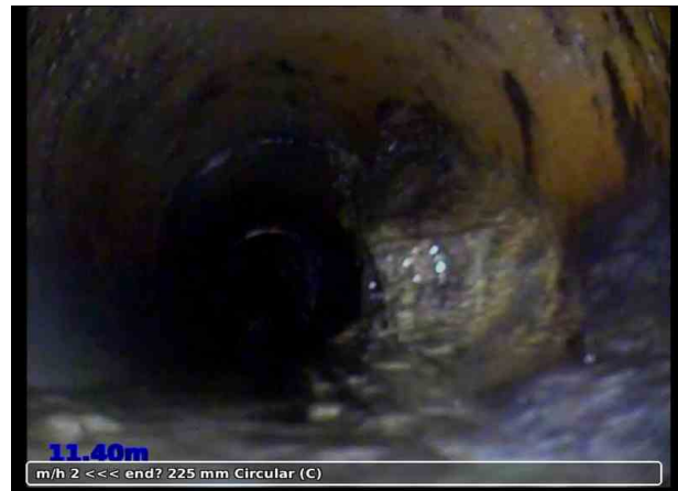
10, 00:01:34, 11.44 m Attached deposits, encrustation from 2 o'clock to 5 o'clock, 10% cross-sectional area loss
