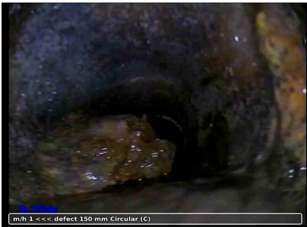
3, 00:01:47, 8.70 m Attached deposits, encrustation from 7 o'clock to 9 o'clock, 20% cross-sectional area loss
