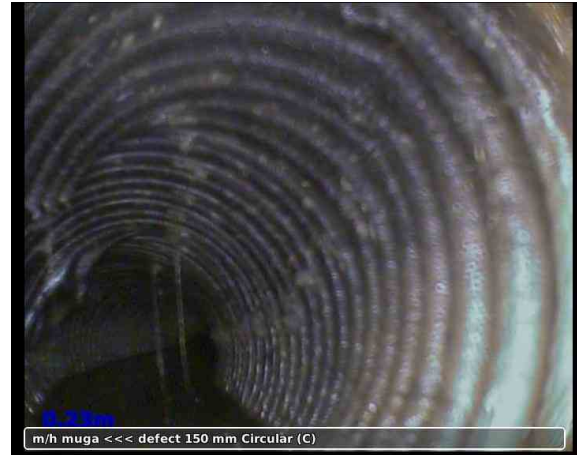
2, 00:00:26, 0.23 m Pipe material changes to an unidentified type of plastic at this point
