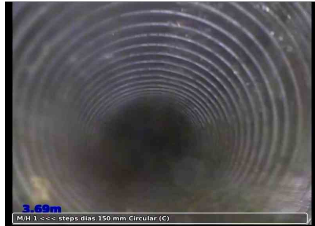
2, 00:03:36, 3.69 m Settled deposits, fine, 5% cross-sectional area loss, start
