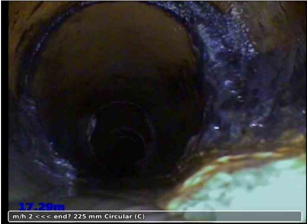
13, 00:00:56, 17.29 m Attached deposits, encrustation from 4 o'clock to 6 o'clock, 5% cross-sectional area loss
