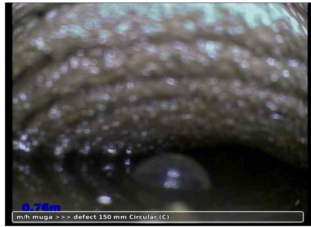
4, 00:01:45, 0.76 m Deformed sewer or drain, 25%
