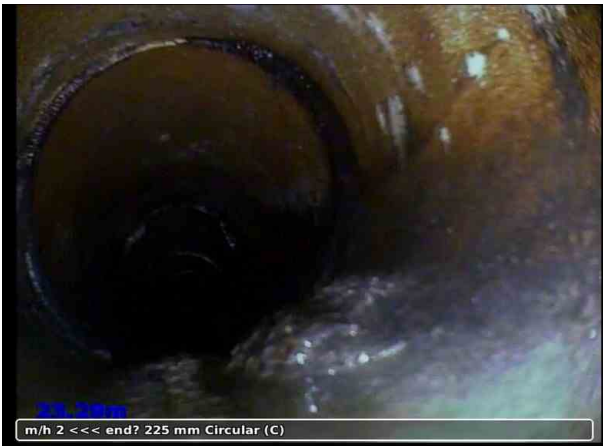
17, 00:00:24, 23.29 m Attached deposits, encrustation from 4 o'clock to 6 o'clock, 5% cross-sectional area loss
