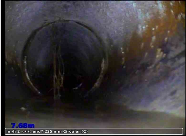
7, 00:01:55, 7.68 m Roots, fine at joint
