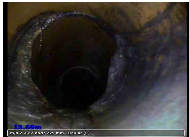
12, 00:01:04, 15.69 m Attached deposits, encrustation from 2 o'clock to 11 o'clock, 5% cross-sectional area loss
