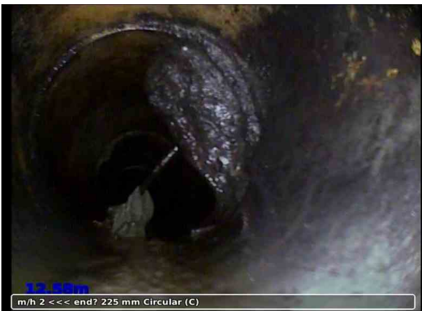
11, 00:01:29, 12.58 m Attached deposits, encrustation from 1 o'clock to 5 o'clock, 10% cross-sectional area loss
