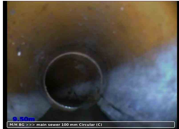
2, 00:01:00, 9.54 m Line deviates left
