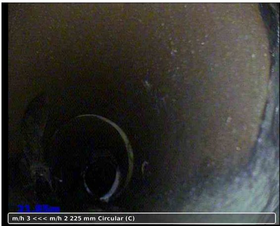
3, 00:00:48, 21.85 m Connection other than junction, at 09 o'clock, diameter: 100 mm
