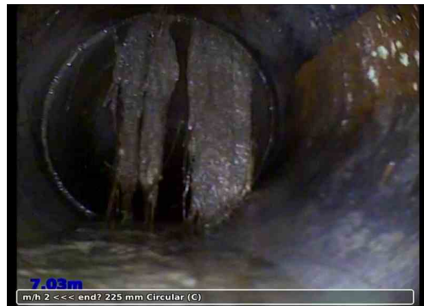
6, 00:02:01, 7.03 m Roots, mass at joint, 25% cross-sectional area loss
