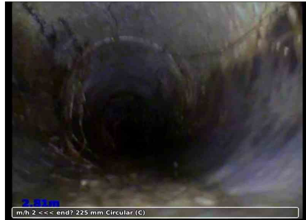
2, 00:02:19, 2.85 m Roots, fine at joint
