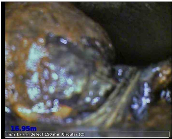
9, 00:00:25, 16.95 m Other obstacles, other object in invert from 5 o'clock to 9 o'clock, 30% cross-sectional area loss
