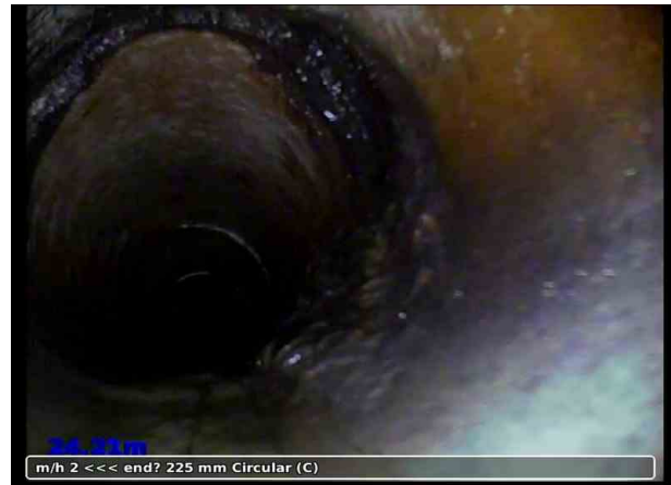
18, 00:00:20, 24.21 m Attached deposits, encrustation from 4 o'clock to 5 o'clock, 5% cross-sectional area loss
