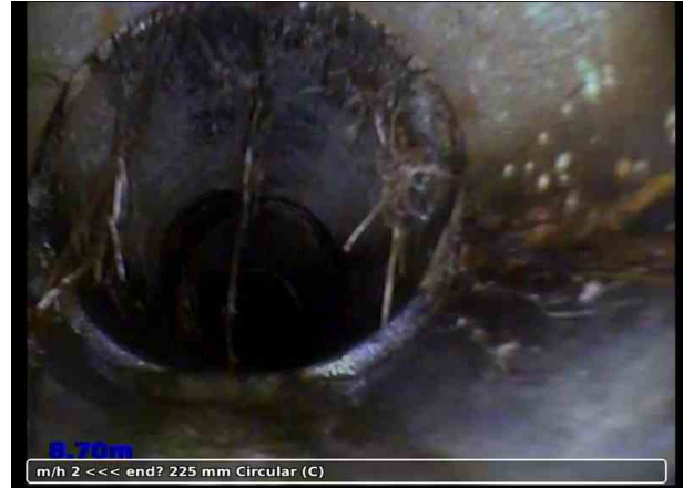
8, 00:01:47, 8.70 m Roots, fine at joint
