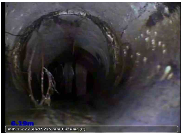
5, 00:02:04, 6.19 m Roots, fine at joint
