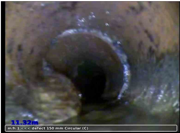
5, 00:01:31, 11.40 m Attached deposits, encrustation from 7 o'clock to 9 o'clock, 10% cross-sectional area loss
