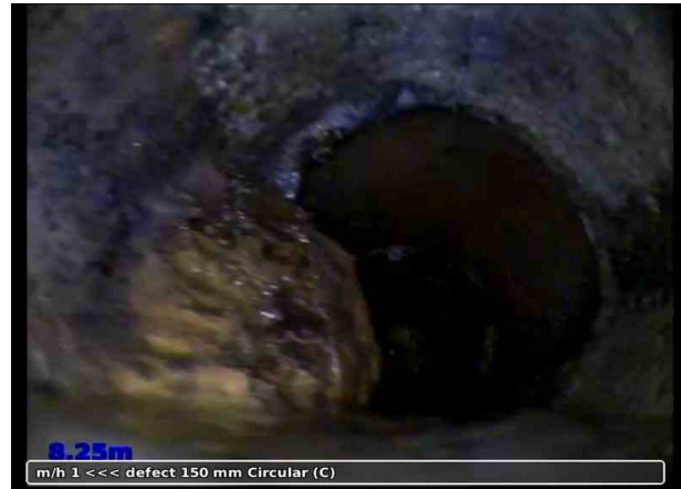
2, 00:01:56, 8.25 m Attached deposits, encrustation from 7 o'clock to 10 o'clock, 5% cross-sectional area loss
