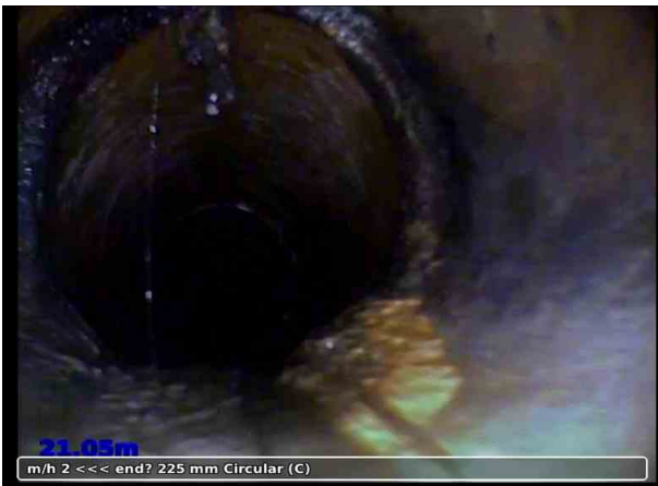
15, 00:00:34, 21.13 m Attached deposits, encrustation at 5 o'clock, 5% cross-sectional area loss
