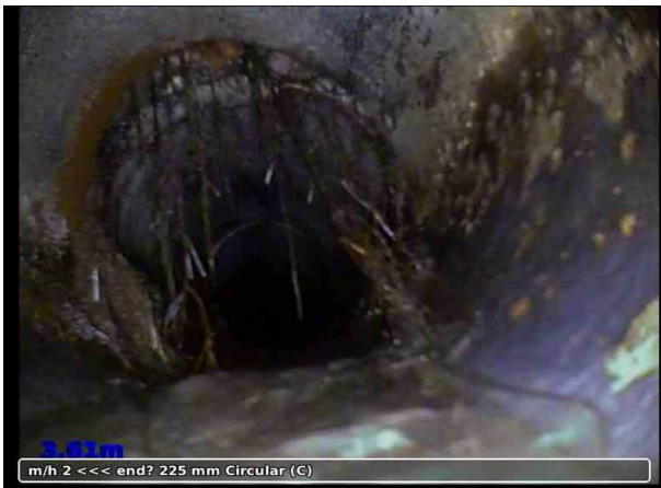
3, 00:02:13, 3.61 m Roots, fine at joint
