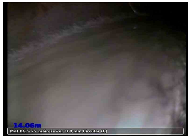
4, 00:00:32, 14.06 m Finish node type, major connection without manhole, reference number: main sewer
