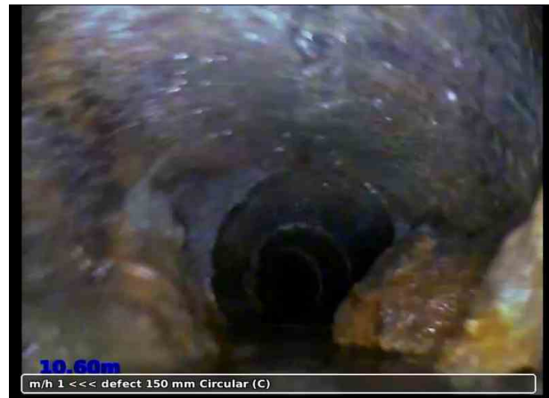
4, 00:01:34, 10.64 m Attached deposits, encrustation from 3 o'clock to 7 o'clock, 15% cross-sectional area loss
