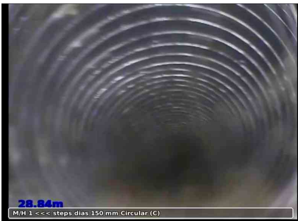
3, 00:01:30, 28.84 m Settled deposits, fine, 5% cross-sectional area loss, start
