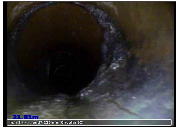
16, 00:00:30, 21.81 m Attached deposits, encrustation from 2 o'clock to 6 o'clock, 5% cross-sectional area loss
