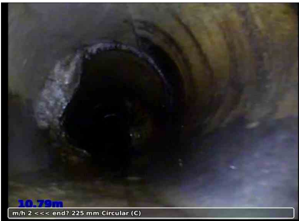
9, 00:01:38, 10.87 m Attached deposits, encrustation from 8 o'clock to 11 o'clock, 5% cross-sectional area loss
