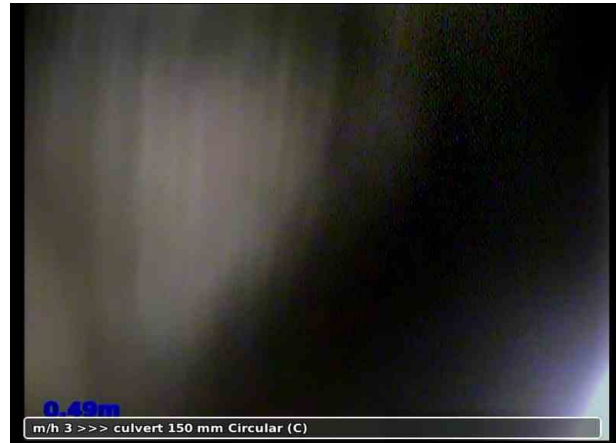
2, 00:00:45, 0.49 m Pipe material changes to masonry (randomly coursed) at this point
