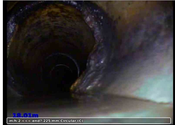
14, 00:00:46, 18.05 m Attached deposits, encrustation from 3 o'clock to 5 o'clock, 5% cross-sectional area loss
